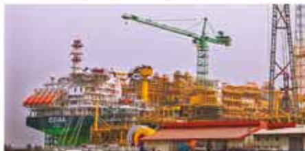
The $3.3bn EGINA FPSO during its modular fabrication at LADOL FZ, Tarkwa Bay, Lagos.
